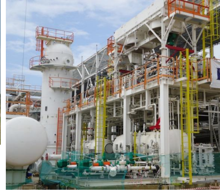
Skid at site
